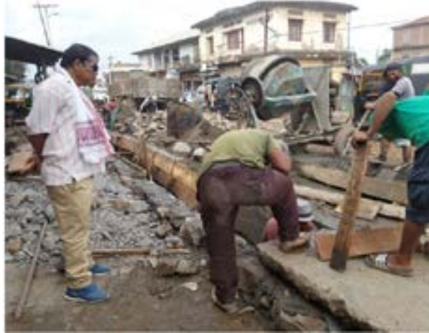
chiapi theilo maleh tuni tiang ah Singngat tiang Water Bound Macadam (WBM) sunsuak a hitai. Nullah hawilo ziak ah lamlian hawitheilo hi ah a kigena, Hmui Veng, Tedim road ah lampi siam thakna nasep ahileh August 27, 2018 ni ah tipper 7, Road Roller leh Grader Machine mang ah kisiam pan a hi. Gua zuk lo hunhun ah nasepna kituptak ah chiapi ngal hiding ti'n Special Contractor T. Lala in a gen hi.
